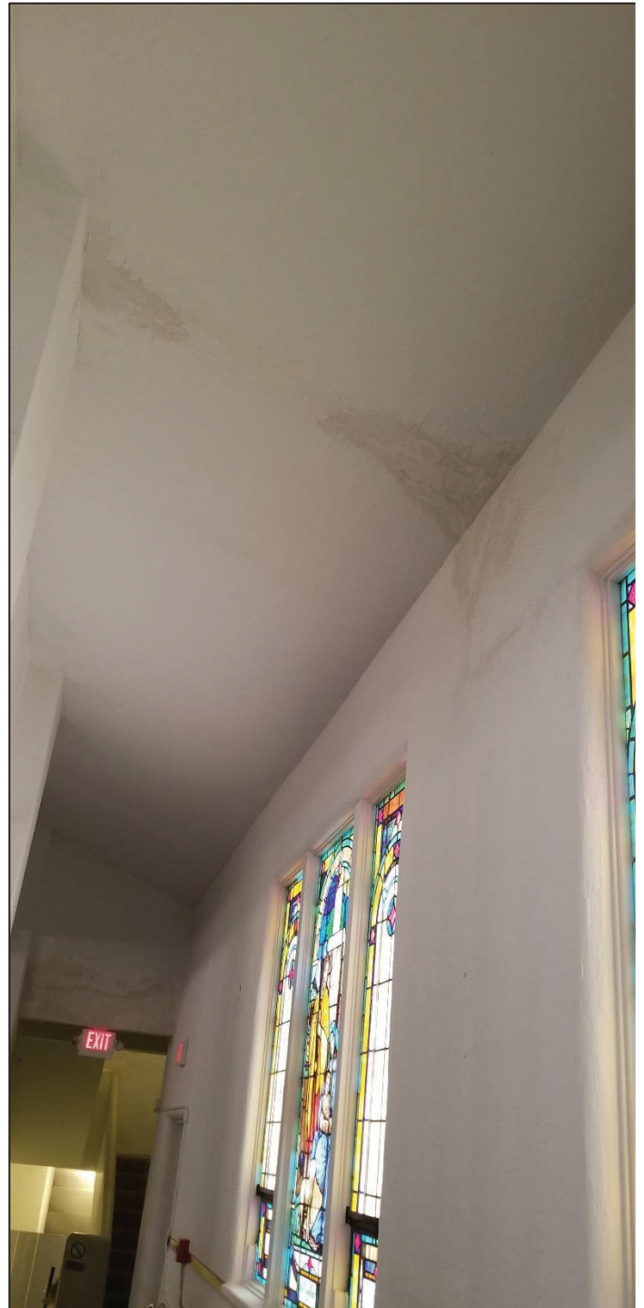
18) Main church main hall, east side lower roof, can be seen extensive water leakage from the roof above.
