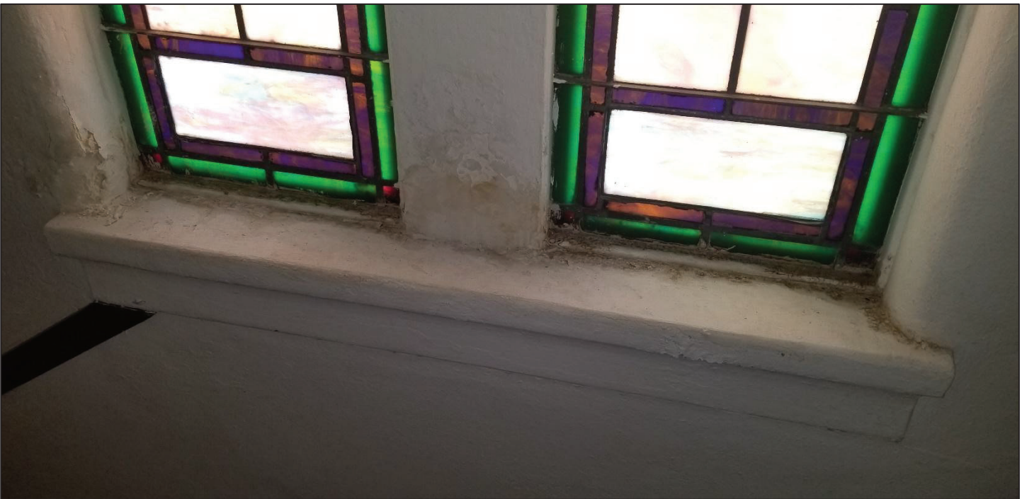
16) Main church main hall, interior fixed windows, south end, can be see moisture stains and peeling all around the window.
