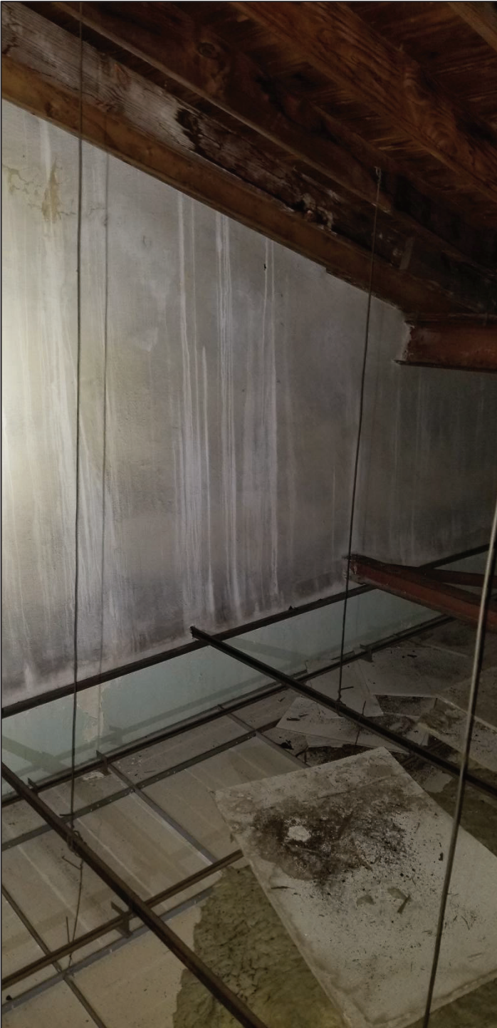
5) Main church, main hall attic space, North end. Can be seen the water streaks that run down from wooden roof diaphragm system above.
