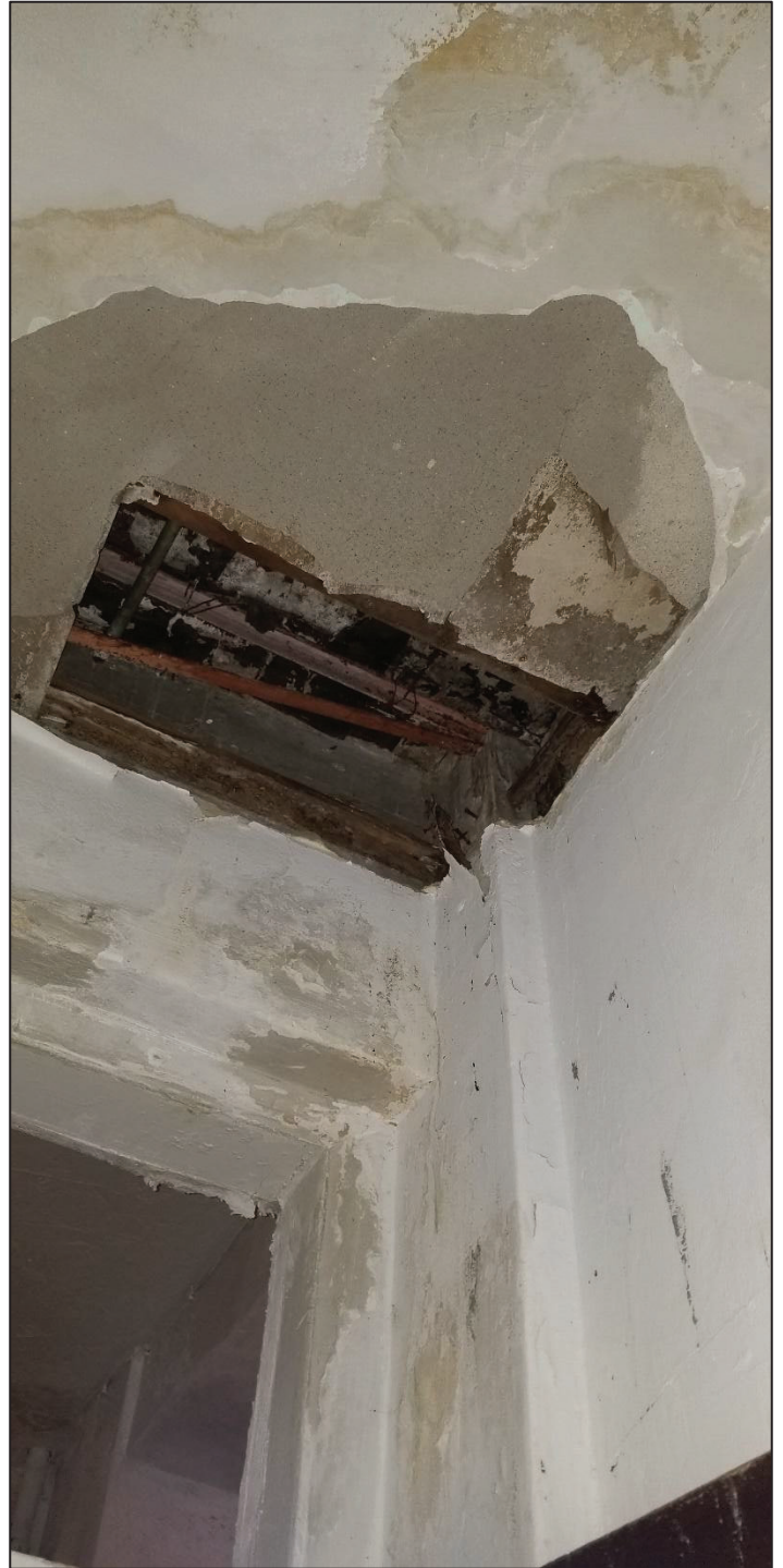
20) Main church main hall, NE side entering the stairway, This part of the ceiling panels collapsed and were later exposed. Can be seen not only the damage to columns and beams around, but also the attic wood members in rotting condition.
