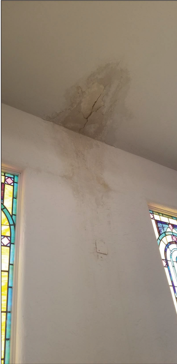
17) Main church main hall, east side lower roof, can be seen extensive water leakage from the roof above.
