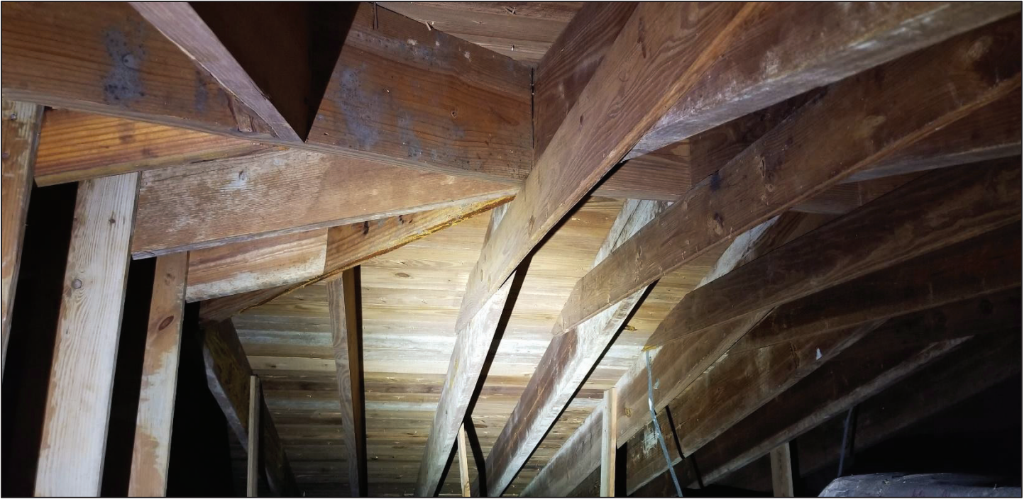
21) Main church, SE structure where offices are located. Can be seen the wood truss members moisture-ridden, at early stages of rot.
