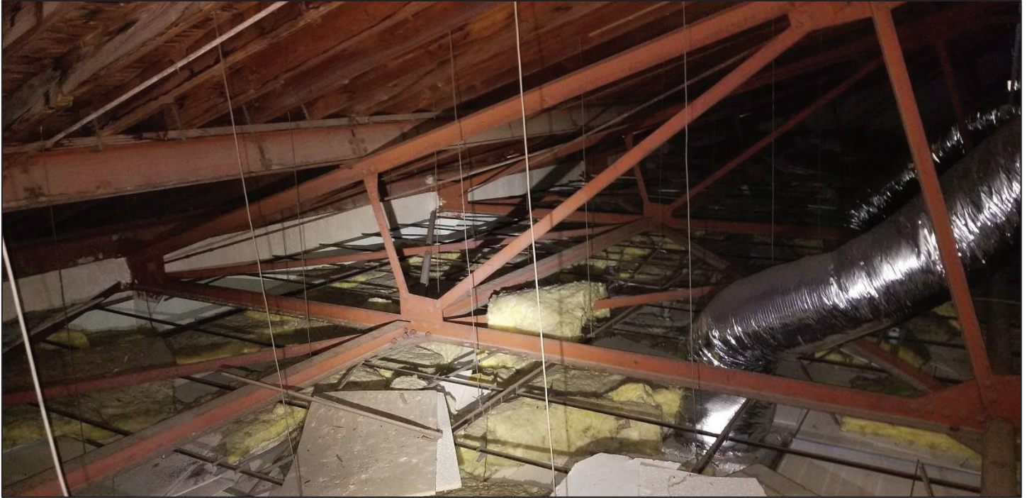
7) Main church, main hall attic space, East direction view. Can be seen steel truss system in good condition but wooden roof diaphragm system above with several moisture-ridden wooden members.
