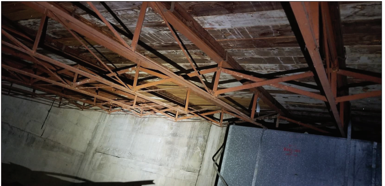
10) Main church, AC unit attic space north region roof system. Can be seen the water streaks that run down from wooden roof diaphragm system above, wood planks from the roof diaphragm above that are moisture-ridden (early stages of wood-rot). The steel trusses are in good condition.
