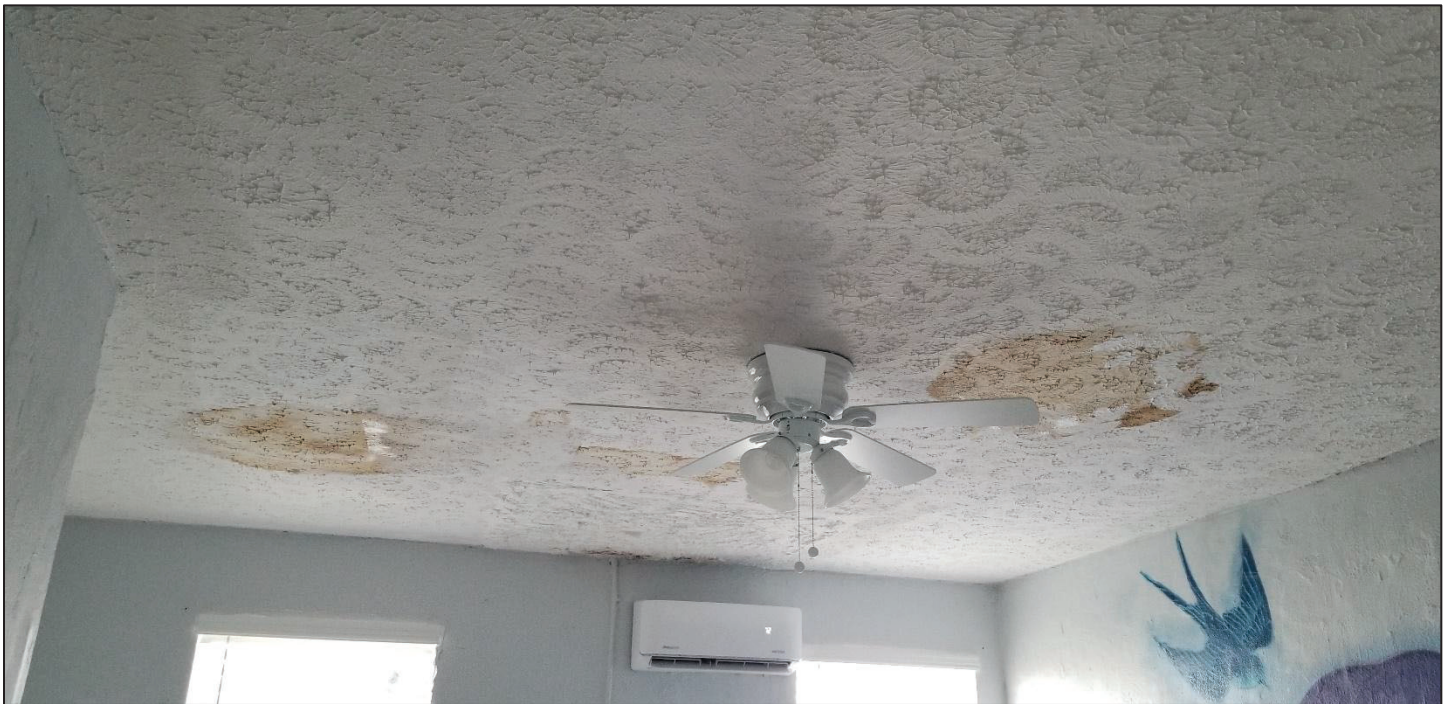
26) Smaller adjacent structure, 2 nd story, can be seen extensive ceiling water stains.
