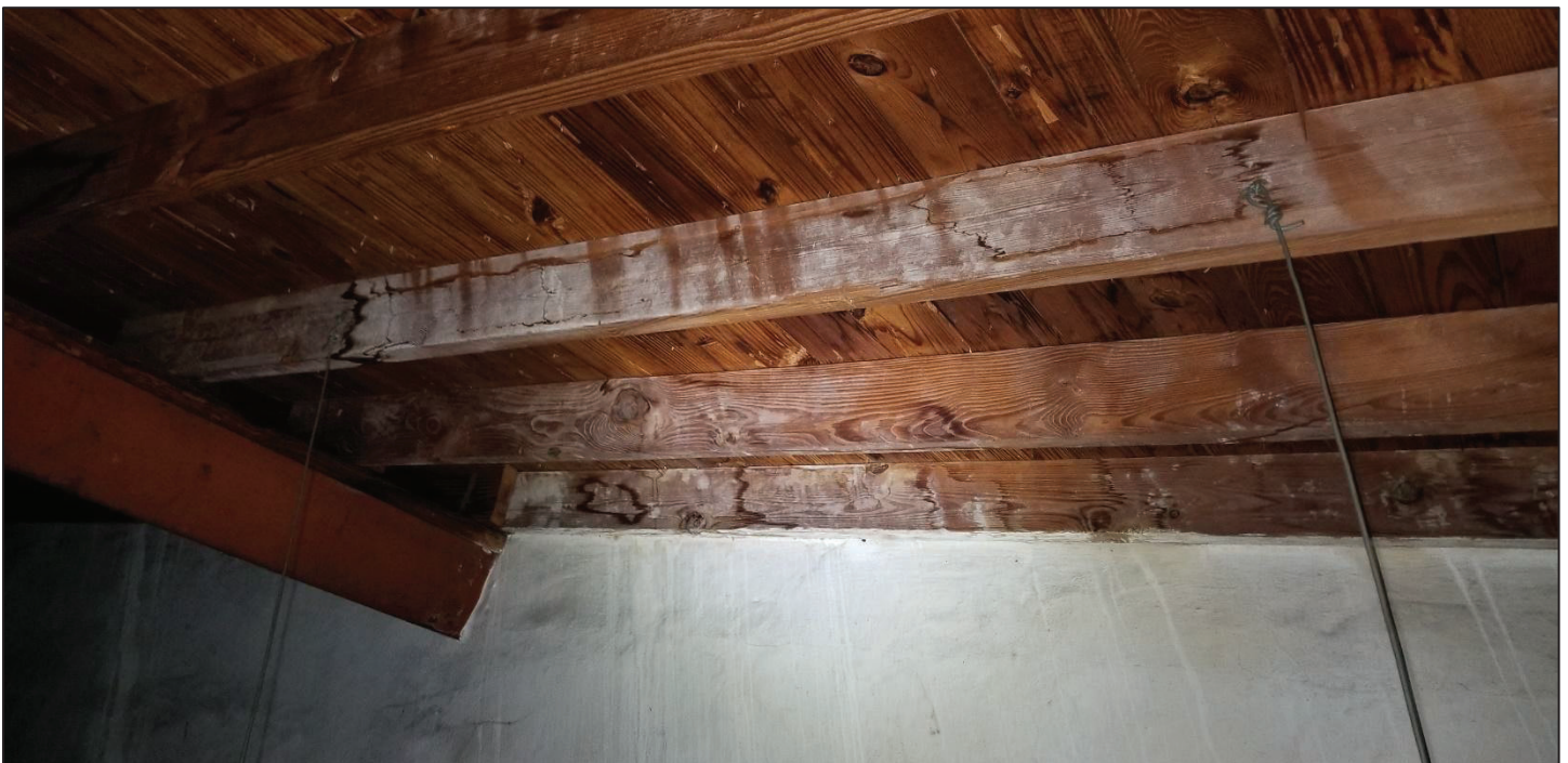
8) Main church, main hall attic space, North end view. Can be seen steel the wooden roof diaphragm system above the steel trusses with several moisture-ridden wooden members.
