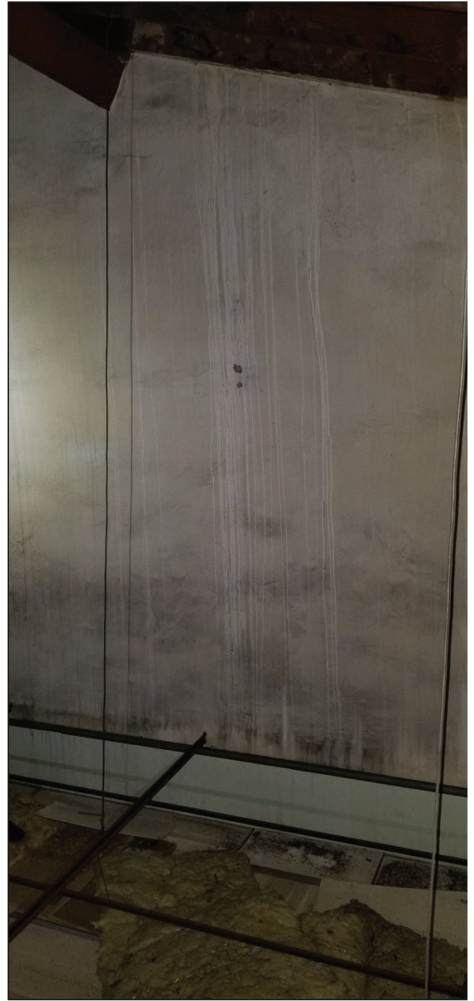
6) Main church, main hall attic space, North end. Can be seen the water streaks that run down from wooden roof diaphragm system above.
