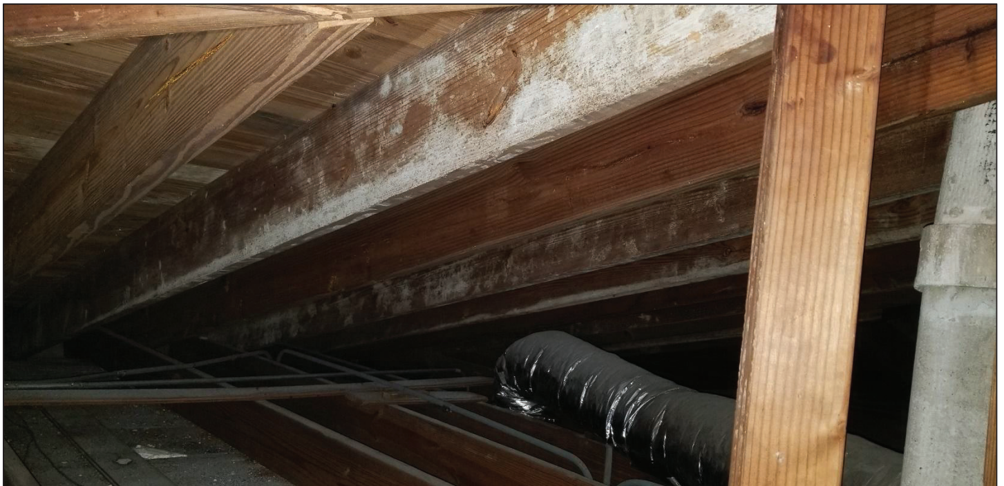
22) Main church, SE structure where offices are located. Can be seen the wood truss members moisture-ridden, at early stages of rot.
