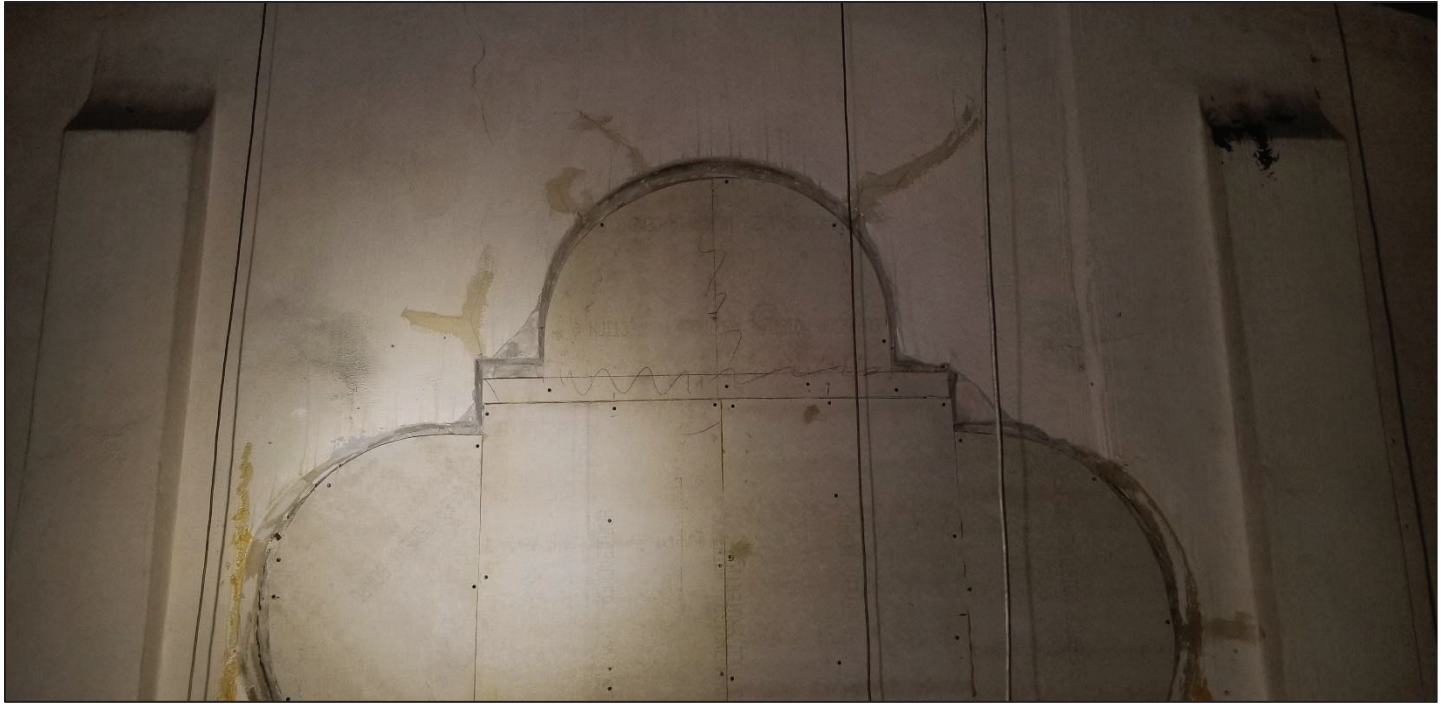
9) Main church, main hall attic space, South end. Can be seen the water streaks that run down from wooden roof diaphragm system above.
