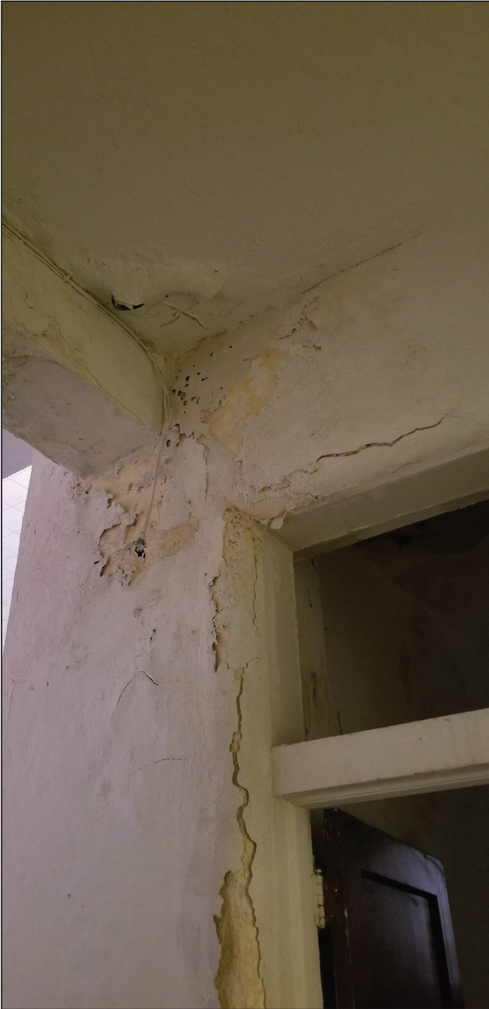
19) Main church main hall, NE side entering the stairway, can be seen much column and beam deterioration due to water and moisture.
